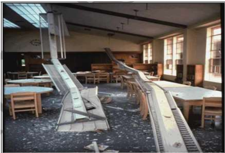
Image 6 – School Damage from May 1983 Coalinga Earthquake ( http://www.smate.wvu.edu/teched/geology/eq-CA-central.html )
