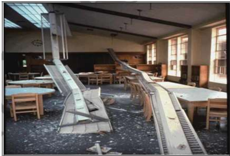
Image 6 – School Damage from May 1983 Coalinga Earthquake ( http://www.smate.wvu.edu/teched/geology/eq-CA-central.html )
